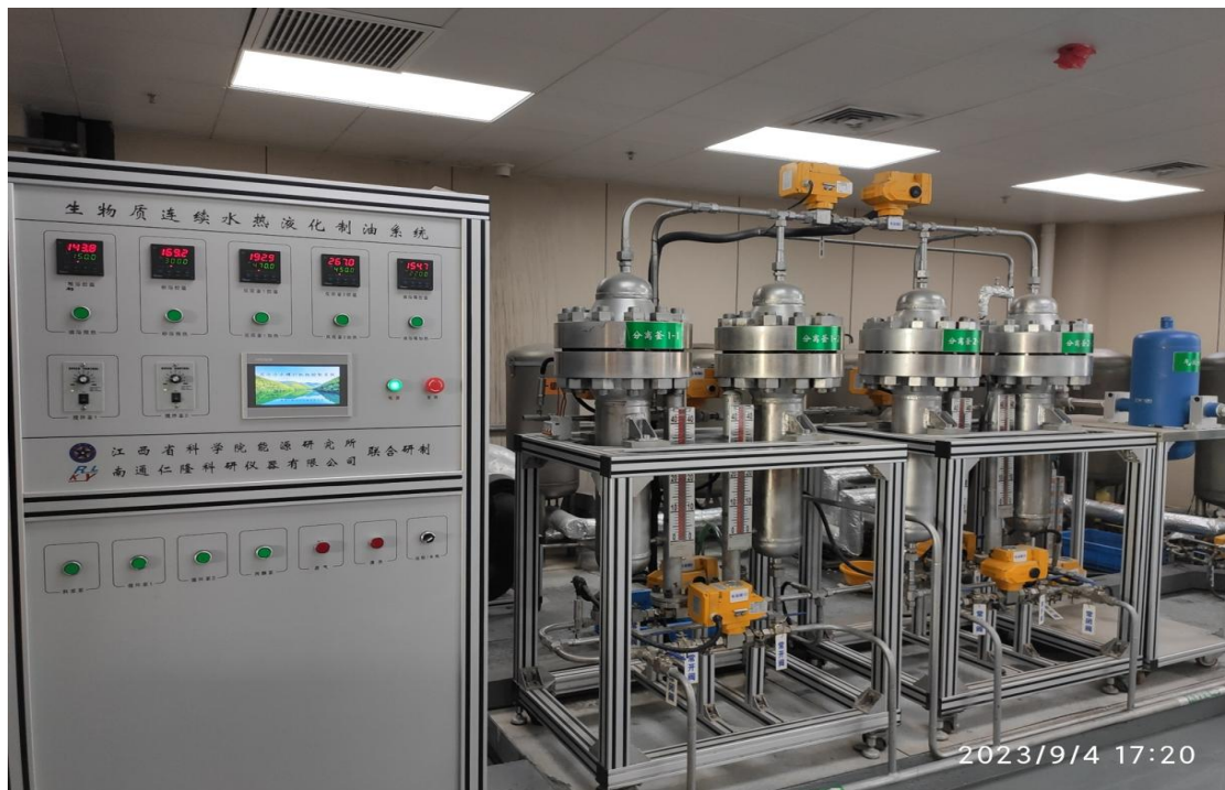
Fig. 2 100 kg/h pilot HTL facility
